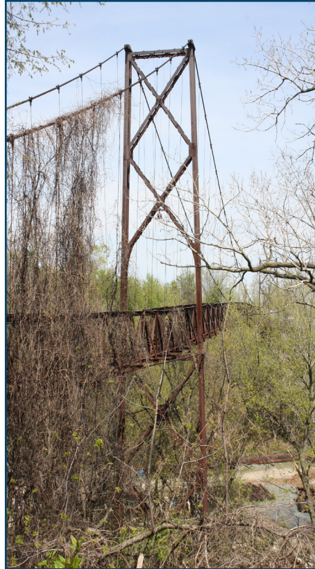
SIDAWAY BRIDGE, CLEVELAND, LISTED IN THE NATIONAL REGISTER OF HISTORIC PLACES IN 2022.
