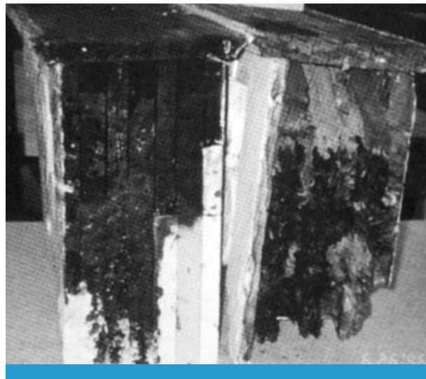
Before and after views of a deteriorated bracket. The bracket on the left was repaired through the use of consolidating epoxy as well as dutchmen.
