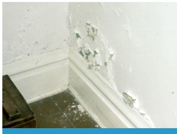
Typical plaster damage that can occur inside a building
