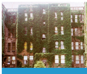
Ivy has overpowered this masonry building
