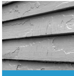
A poorly prepared paint surface. Note how the edges of the scraped sections have not been feathered.
