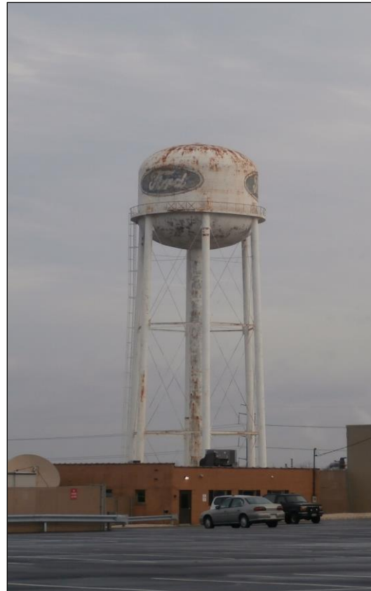
Plate 25. Water tower at the Ford Stamping Plant in Walton Hills taken November 2016.
