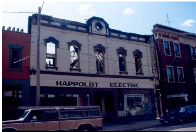
ALL THAT REMAINS OF THIS BUILDING AFTER A DEVASTATING FIRE IS THE FAÇADE. HOWEVER, WITH PROPER EVALUATION AND PLANNING IT MAY BE POSSIBLE TO STABILIZE THE FAÇADE AND CONSTRUCT A NEW BUILDING, WHILE MAINTAINING THE ARCHITECTURAL INTEGRITY OF THE COMMERCIAL DISTRICT.
