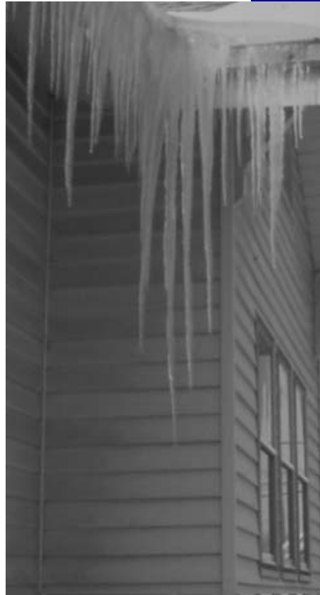
Dangerous icicles that have formed along unheated eaves.
