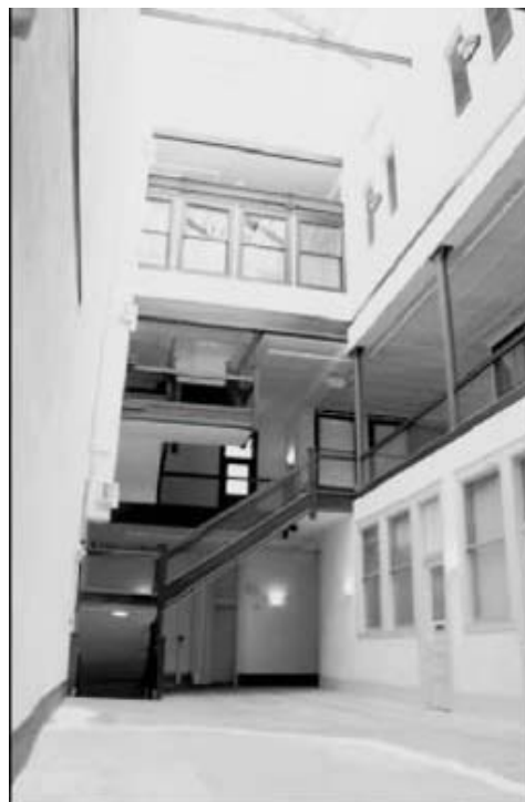
Use of 3410 allowed the retention of an atrium and two open stairs in the Merrell Building rehabilitation in Cleveland.
