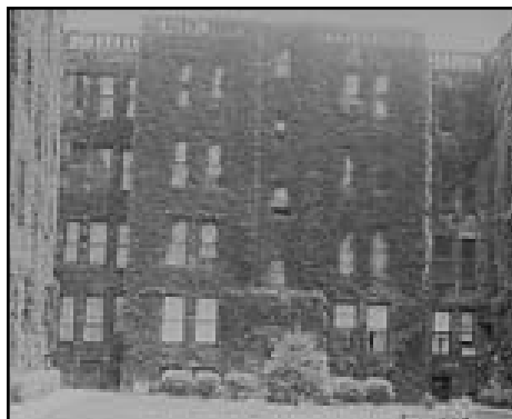
Ivy that has overpowered this masonry building.
